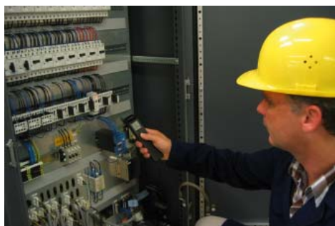
Detailed infrared temperature measurement of an electric control with the help of the installed close focus optics for 1 mm ranges of the optris LS LT
