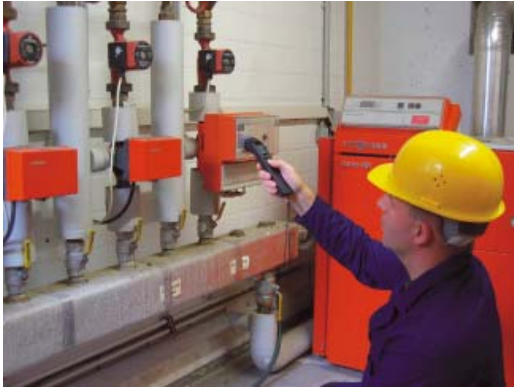
Checking the temperature of heating circles
